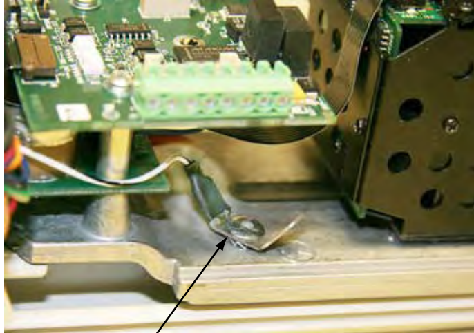
E1 Chassis Ground Ground Lug for Cable Overall Shield (Solder direct or use spade lug)
